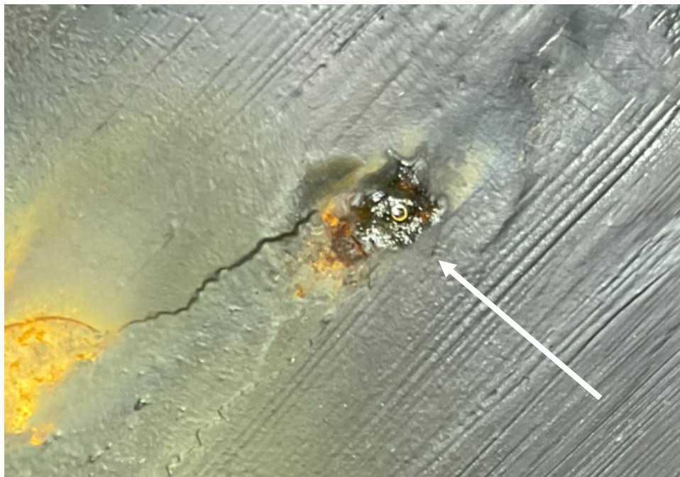
Figure 3.—Example of a pressure tap with corrosion and coating loss causing surface irregularities near the tap.
