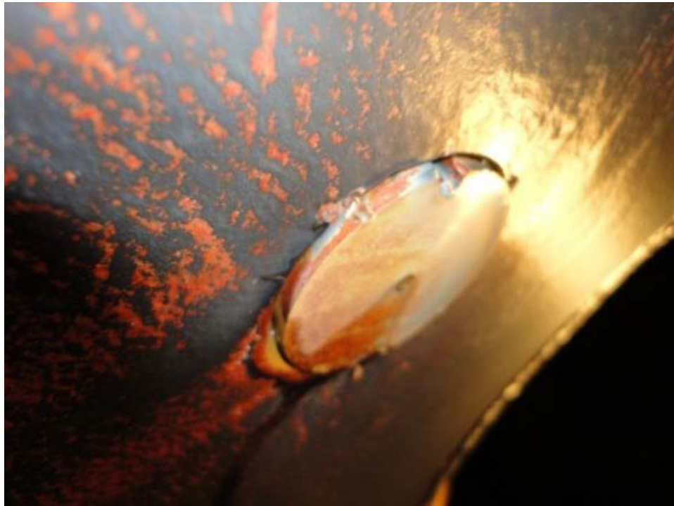
Figure 2.—Example of a pressure tap insert that protrudes inside the pipe wall causing an offset.
